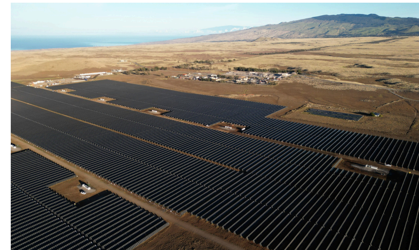
Hale Kuawehi, a 30 MW solar plus battery storage project, came online in March 2025
