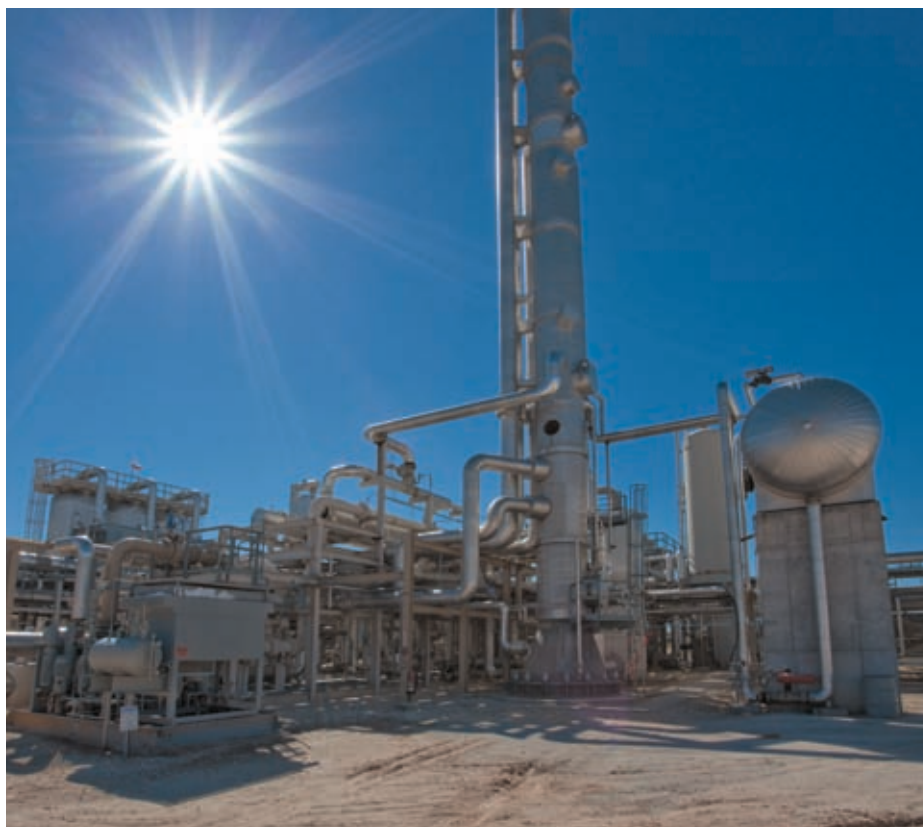
The 200 MMcf/d capacity of the Cowtown processing plant provides highly efficient cryogenic processing for producers extracting more than 90% of the ethane from the gas stream.
