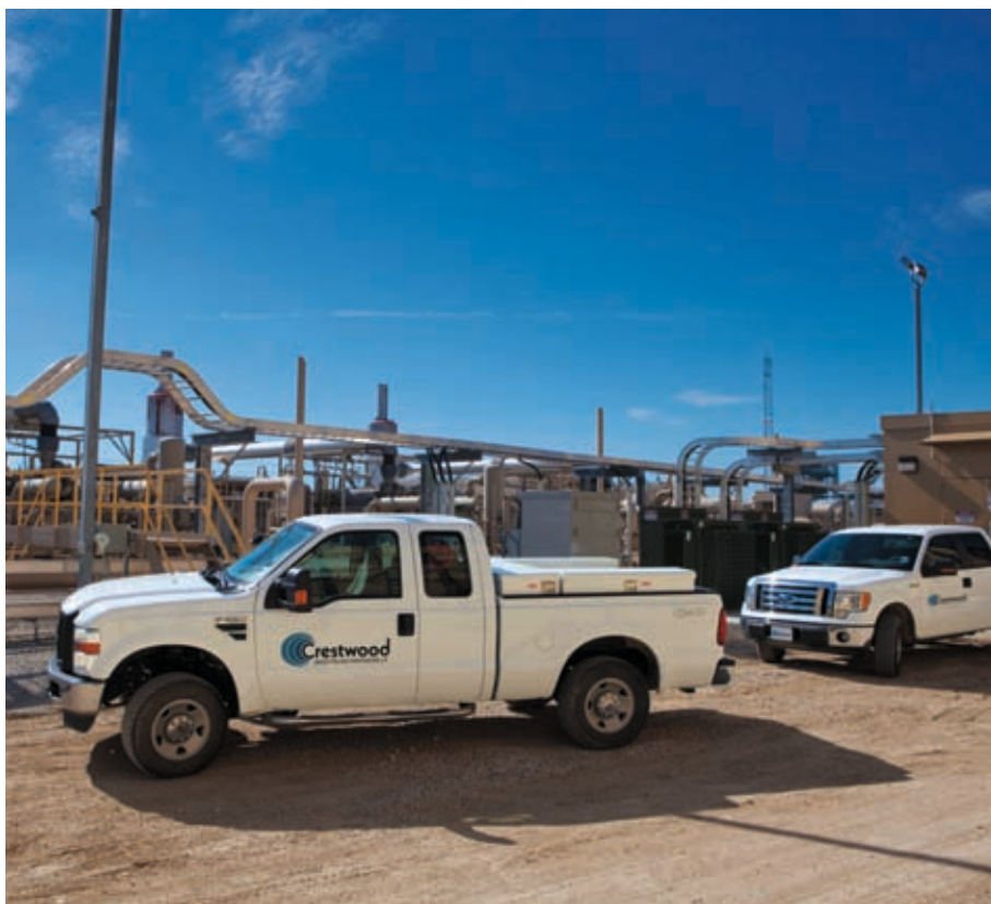
The Lake Arlington Station includes three electric-driven compressors that provide efficient and reliable service with lower noise emission in the Fort Worth metropolitan area.
