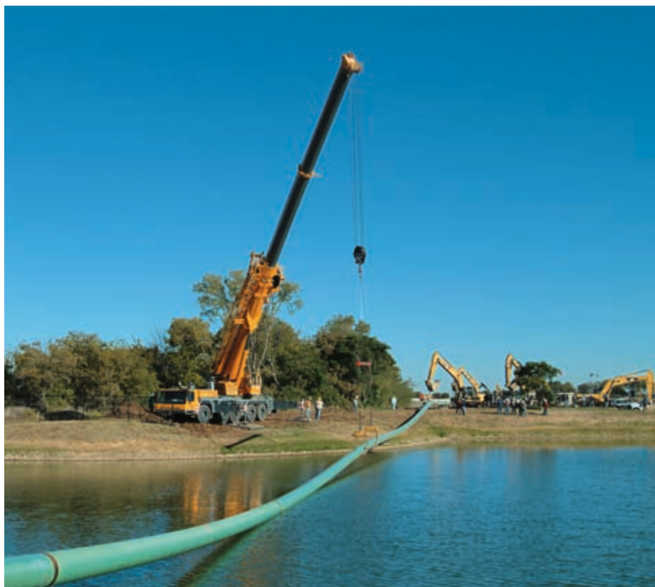
During 2010, Crestwood continued to expand the gathering capacity of the Alliance system. Here gathering pipeline is being staged for a nearby directional bore.
