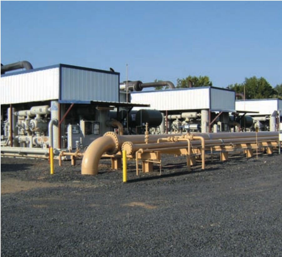
The Fayetteville Shale Woolly Hollow station, constructed in 2010, includes 10,650 HP of compression and treating capacity of 60 MMcf/d.
