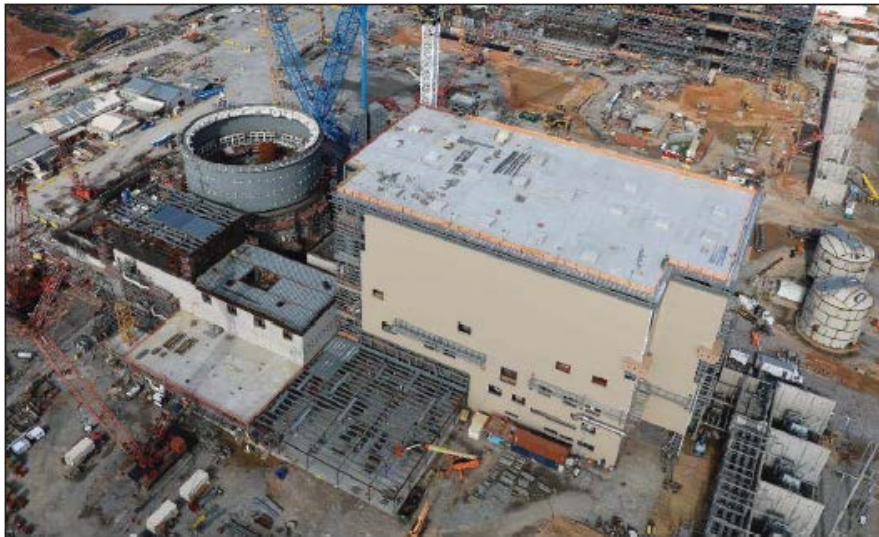
Unit 3 Nuclear and Turbine Islands
