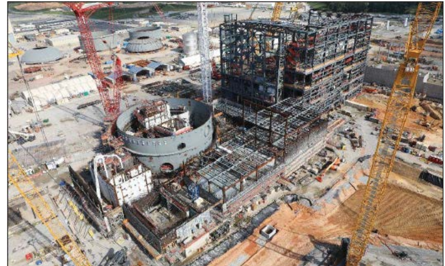
Unit 4 Nuclear and Turbine Islands
