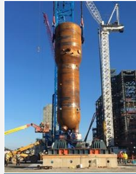
Unit 4 Steam Generator (A)
