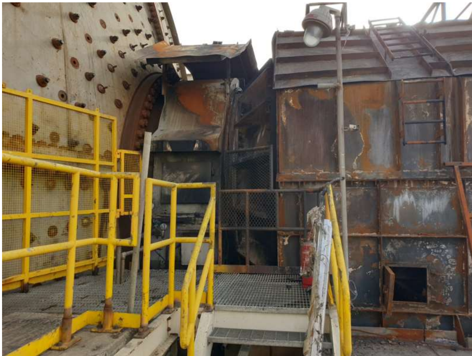
Figure 3: SAG mill discharge trunnion bearing and trommel
