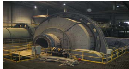
SAG Mill installed at site
