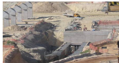
Stockpile area: base and the conveyor tunnel to feed the SAG mill
