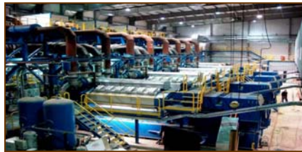
Wartsila generators installed at site
