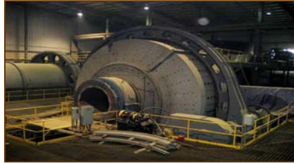
SAG Mill installed at site
