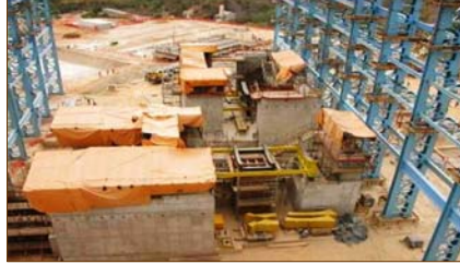
SAG and ball mill progress: October 2007
