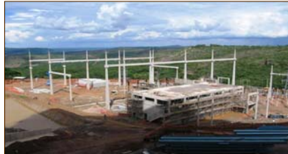
Main substation: December 2007
