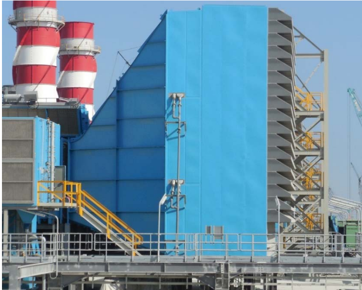
Gas turbine filters
