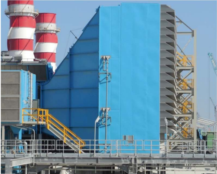
Gas turbine filters
