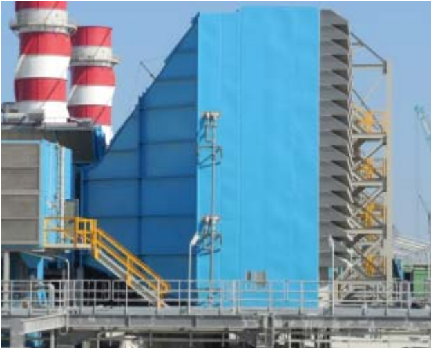
Gas turbine filters
