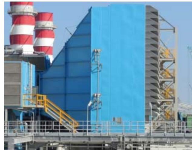
Gas Turbine Filters
